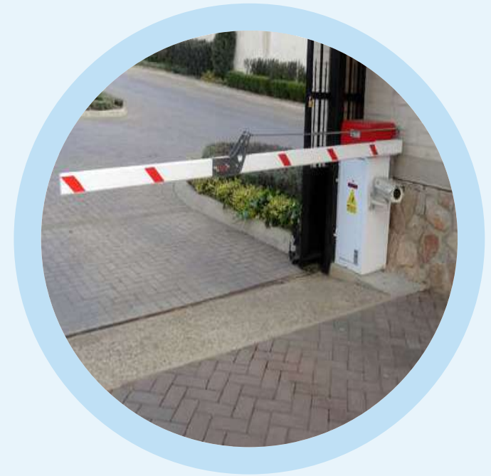
BOOM BARRIER SYSTEM
